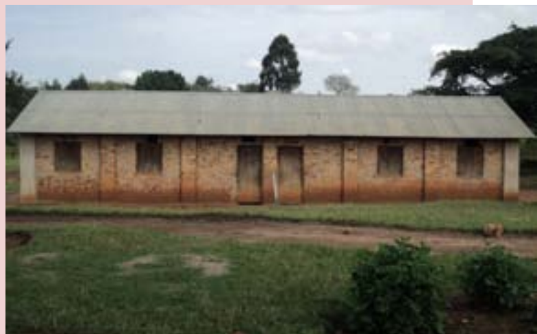
A two classroom block at Mpara primary school put up by parents but left incomplete due to inadequate capacity.
