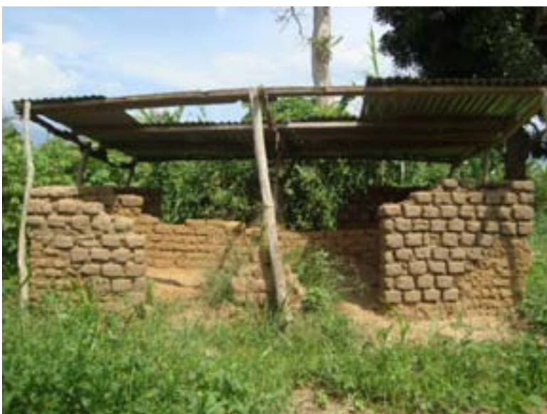
A pit latrine (shared by both pupils and teachers) at Bundimbela Primary school in Bundibudgyo.
